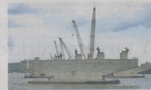
PETER CARR/THE JOURNAL NEWS Workers stand on a concrete support pier as they wait for a girder assembly to be set in place for the new Tappan Zee Bridge in June.
